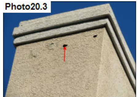
Holes need to be sealed
