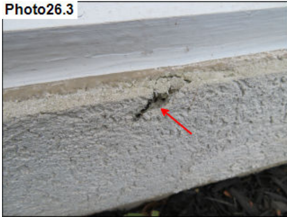
Damage typical where noted in the report
