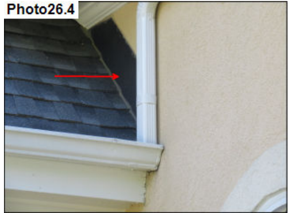
Counter flashing is installed instead of a kickout flashing
