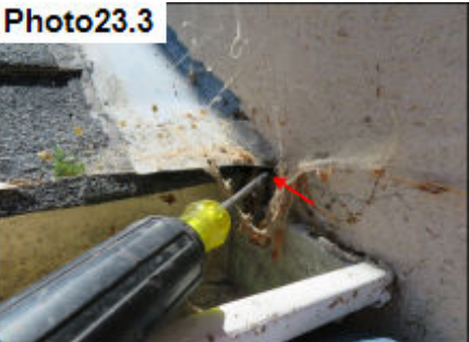
Gap under flashing & gutter
