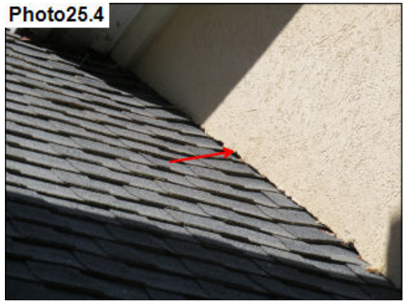
The EIFS runs to the shingles in some areas
