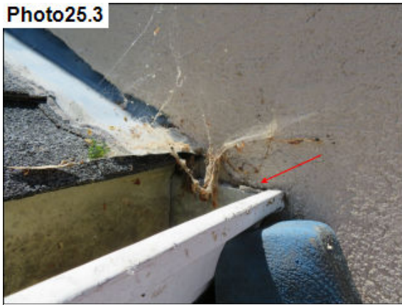
Kickouts are not installed
