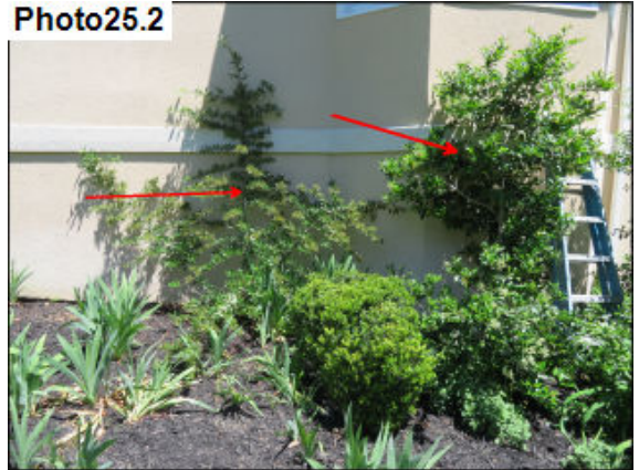
Keep shrubbery cut back off house 18 to 24 inches.
