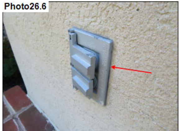
Outlets are sealed
