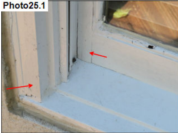
Wood rot at windows
