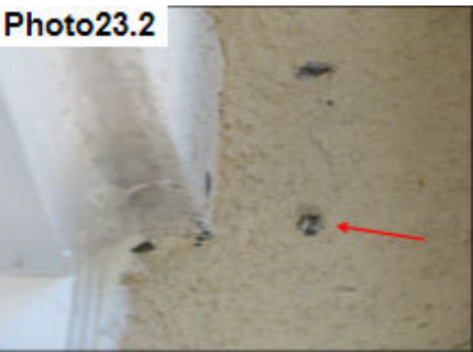
Holes need to be sealed
