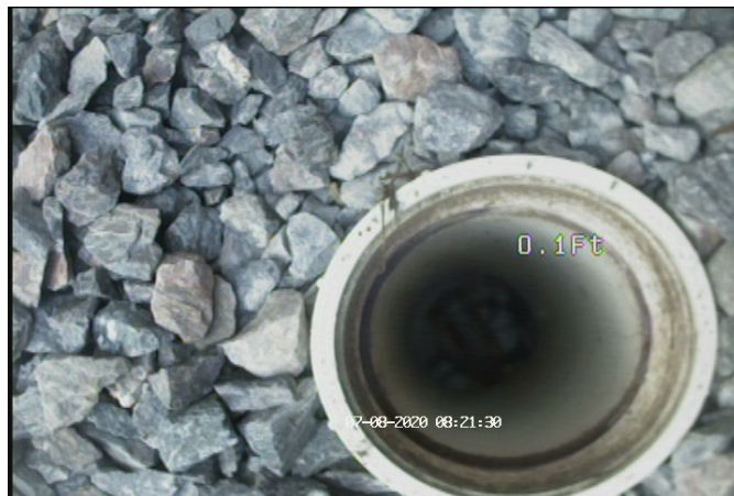
Entry point from cleanout by rear of the home
